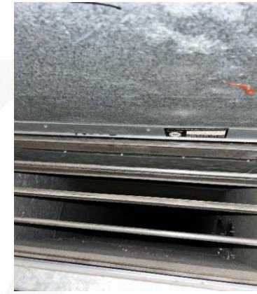
Photo of Damper as Left
