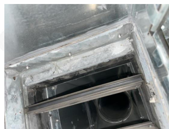
Photo of Damper as Left
