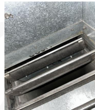
Photo of Damper as Left
