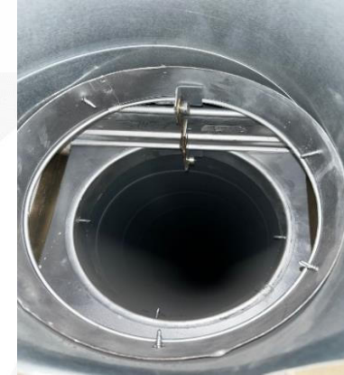
Photo of Damper as Left
