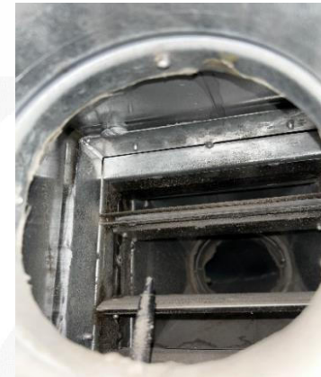
Photo of Damper as Left
