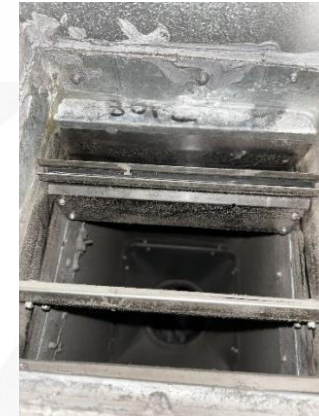
Photo of Damper as Left
